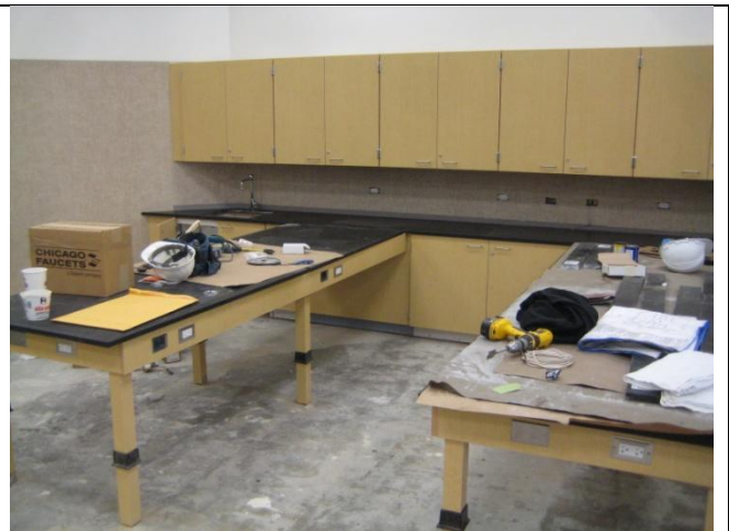
Epoxy counters and wallpaneling in the labs
